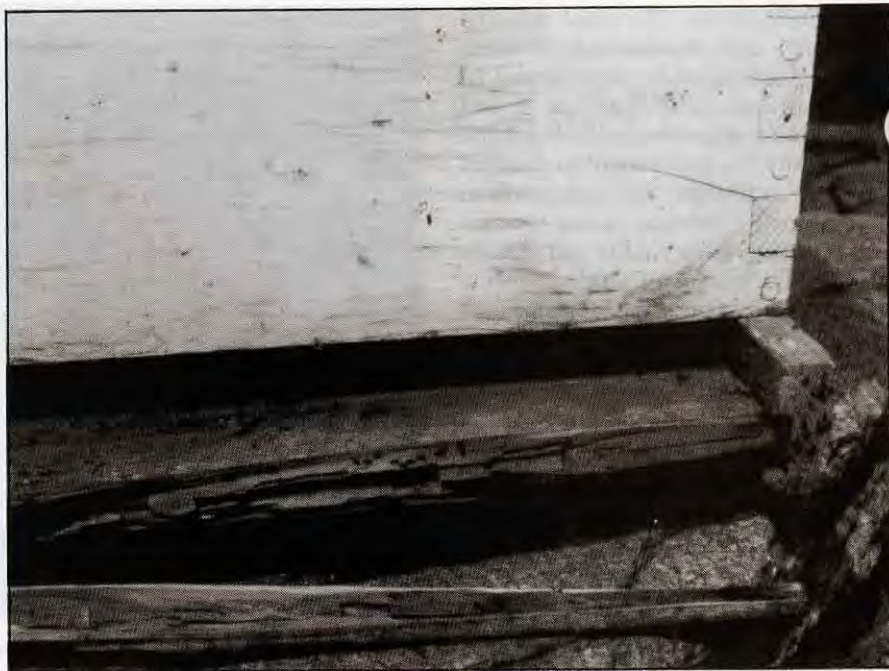
Although this bottom was once painted, it was neglected as it aged. Weather and insects were able to attack from underneath as well as through the joints.
