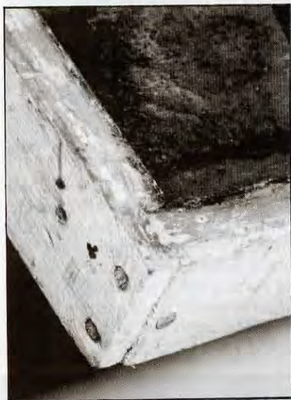
Standing water on landing platform can seep into the joints, even in a well constructed bottom board. This one is still sound. It has been kept painted.
