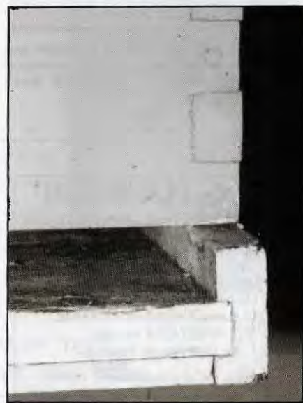
This bottom board is old, but it is still sound. All the surfaces of the rabbet joint were painted for assembly.
