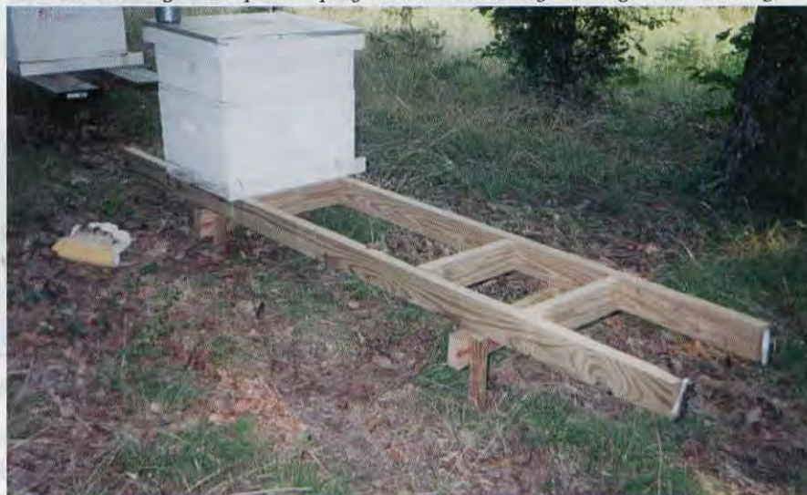
Detail showing how top 2 x 4 platform is constructed for strength and stability.
